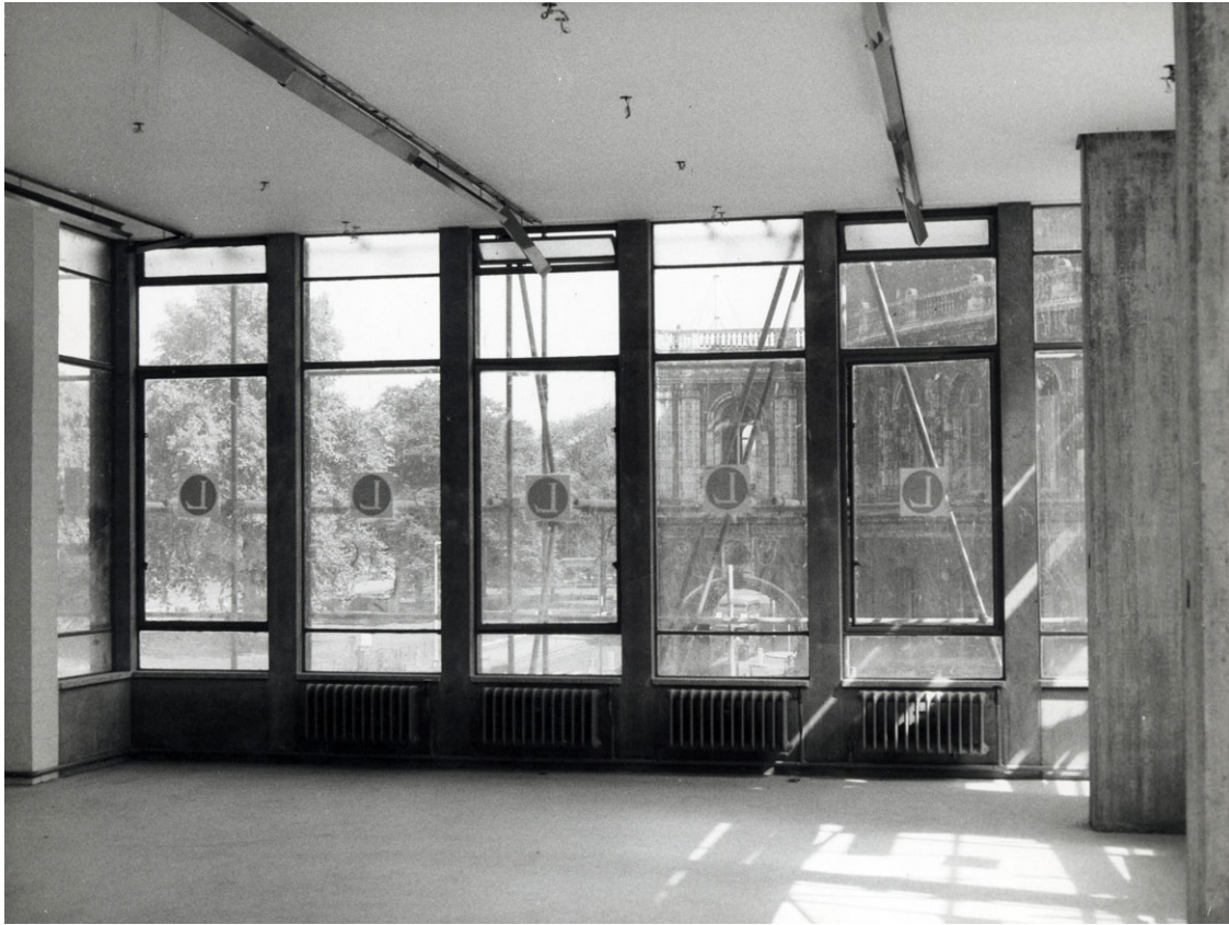
Figure 4. Construction of the Royal College of Art Workshop block (later known as Darwin Building). Courtesy Royal College of Art archive; photographer unknown.
