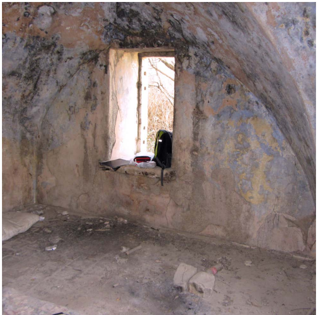
Figure 11. House 62, missing protection bars. Courtesy of Riwaq Centre: Lifta documentation project.
