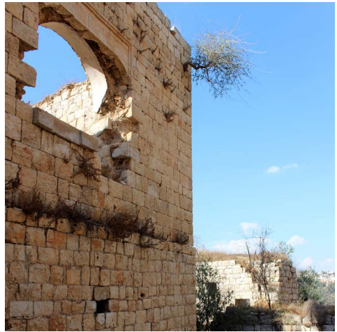
Figure 13a. House 28, missing window. Courtesy of Riwaq Centre: Lifta documentation project.
