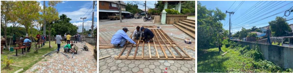
Figure 29: The local administrative staff from the Bureau of Public Works constructed a stair, paved a new walkway along the wall and built a backdrop for the pilot market.
