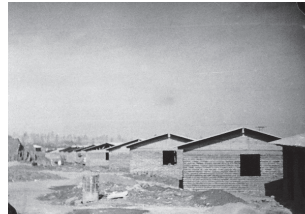
Fig.66 Villa La Reina during construction by the families themselves. Source: Alvarado, 'Auto Construcción', 36.
