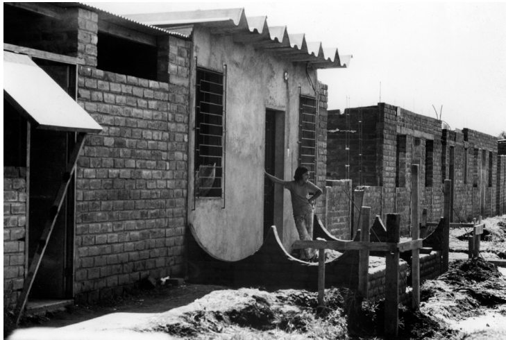
Fig.3 Sites and Services project: core units built in San Salvador, El Salvador, c1975. Source: World Bank Group/ Jaime Martín Escobal.
