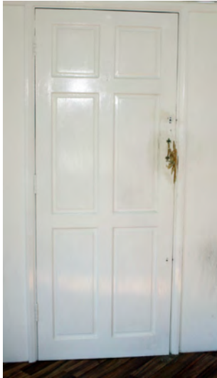
Figure 8. Before: a damaged wall
